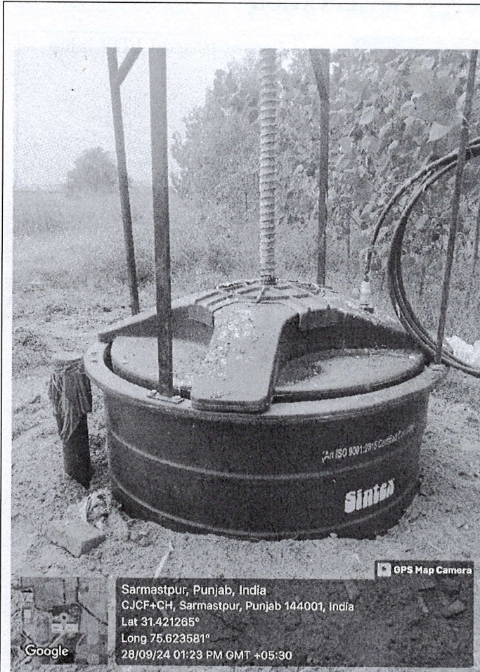
Bio Gas Plant
